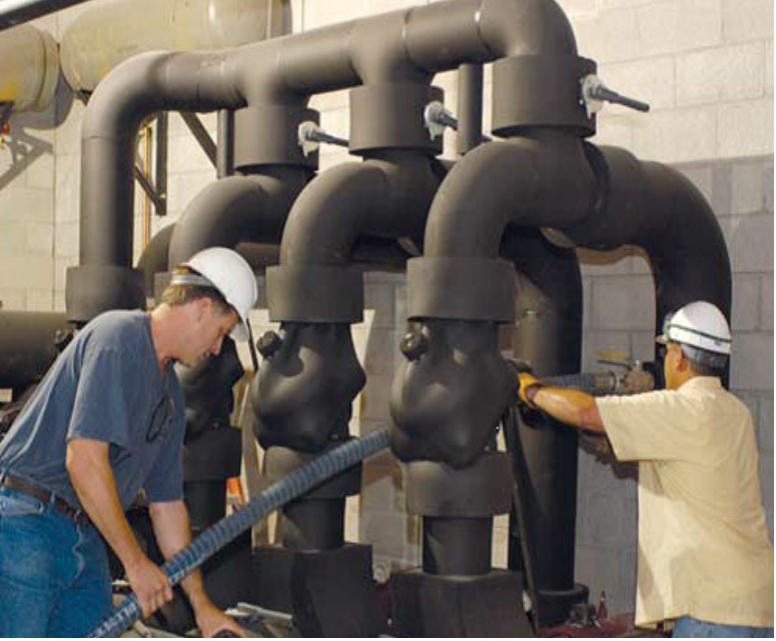
Daniel Laitila of Serve-Ice (left) and truck driver Bernie McClain (right) work together to fill high-performance DOWTHERM™ SR-1 Heat Transfer Fluid into the Midland Civic Arena ice refrigeration system.
