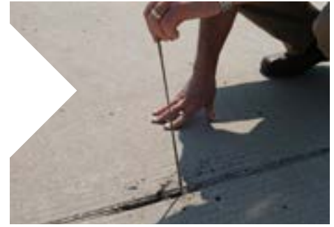
Field adhesion testing identifies issues such as improper joint cleaning, improper sealant installation or other problems that could negatively impact the adhesion of the cured sealant.
